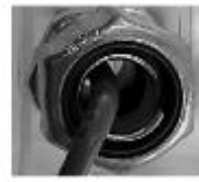
Conduit with Cable
