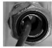
Conduit with Cable
