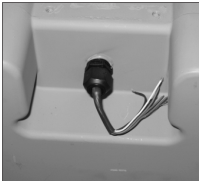
Figure 7.8- Pulse output cable on backside of meter
