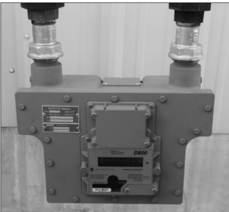
Figure 5.4 -Meter placed in line
