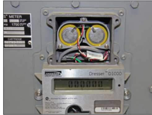
Figure 9.30 Example - Battery pack in place
