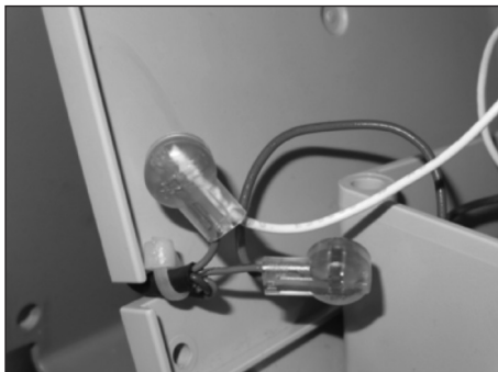
Figure 7.21 Example - ERT cable properly routed through the back plate
