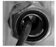
Conduit with Cable
