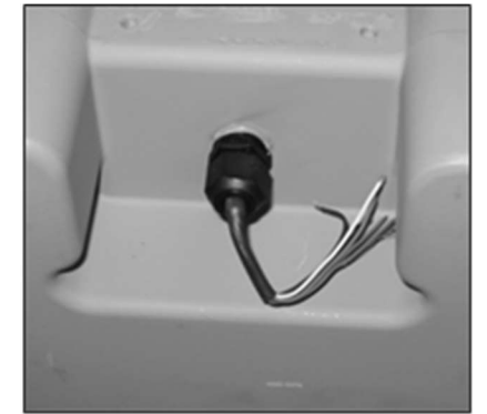
Figure 18: Pulse output cable on backside of meter
