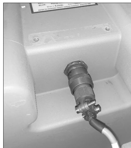
Figure 23: Pulse output cable plugged into connection
