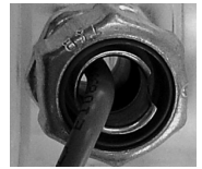
Conduit with Cable
