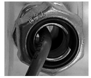
Conduit with Cable
