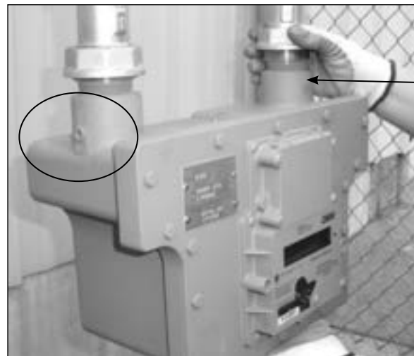
Figure 11.1 Example - Differential pressure taps are located on the inlet and outlet connectors
