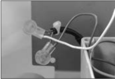
Figure 7.20 Example - Pulse Output 2 wired to the ERT with a cable tie located near the end of the shrink tubing
