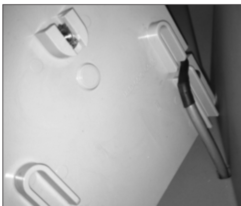
Figure 7.22 Example - Meter cable routed across back plate
