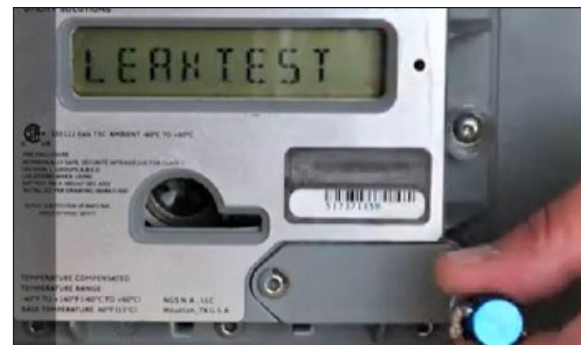
Figure 7.7 Example - Scroll to LEAKTEST screen
