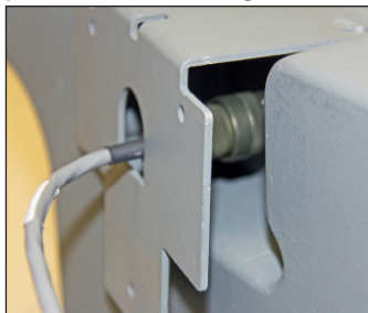
Figure 7.28 Example - Pulse output cable is covered by a protective plate
